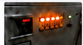
Testing, Commissioning & PF Fine-Tuning
