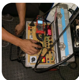
Protection Relay Test
