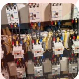
Replacement Contactor & MCCB
