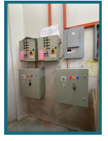
Unit 3 & 4 - Main Switch Room
